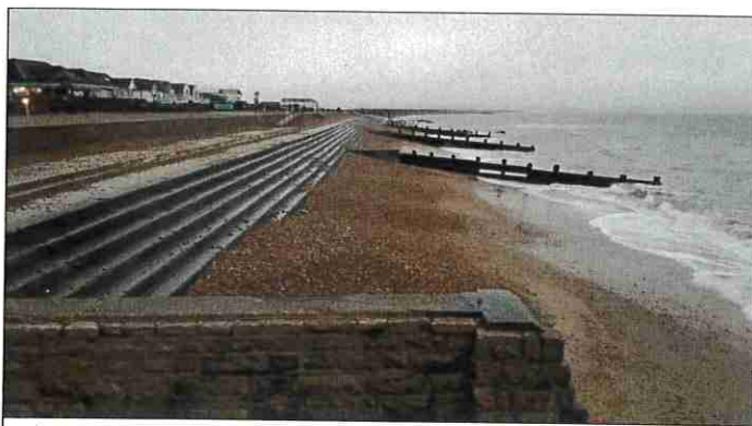
Timber groynes to the east of the new beach huts at Milford on Sea are damaged, suffering loss of planks. Storm Eunice, February 2022
